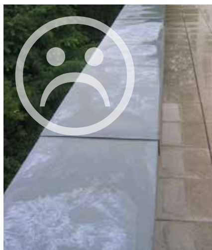
Zinc hydroxide formation due to insufficient slope
